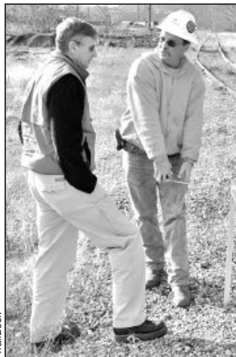
Trail Coordinator Jack Paulik (left) and Roger "Bucky" Walker, P.J. Dick/Trumbull construction foreman, discuss trail grading.
