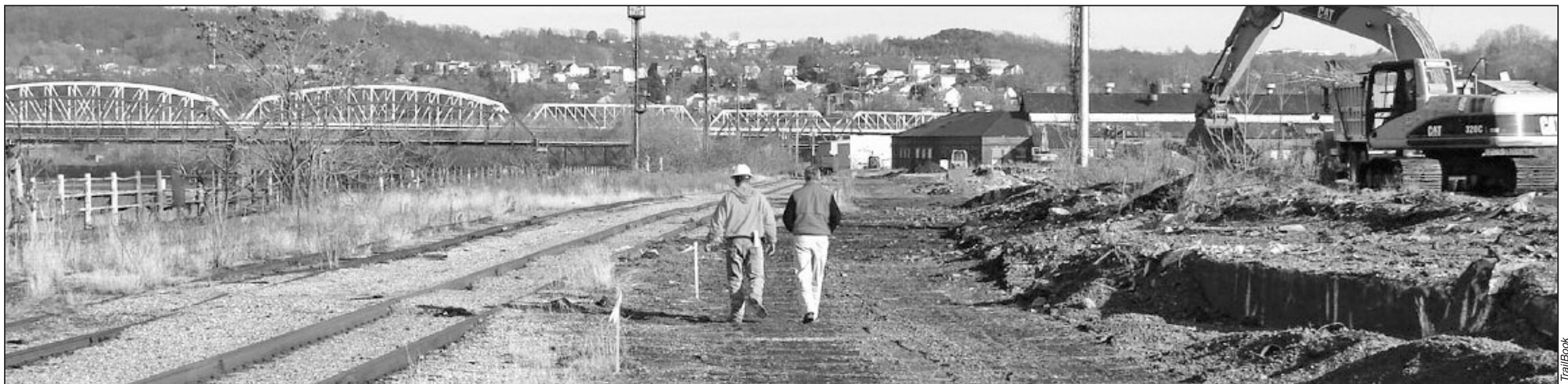
Grading begins along the Monongahela River in McKeesport in what was once the National Tube Works of U.S. Steel. The trail will cross the river on the Riverton Bridge visible in the background in front of the lighter Duquesne-McKeesport Bridge.
